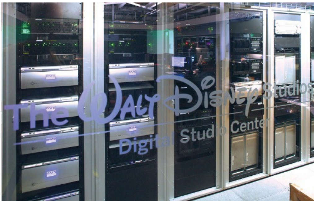
Digital Media Center Machine Room
