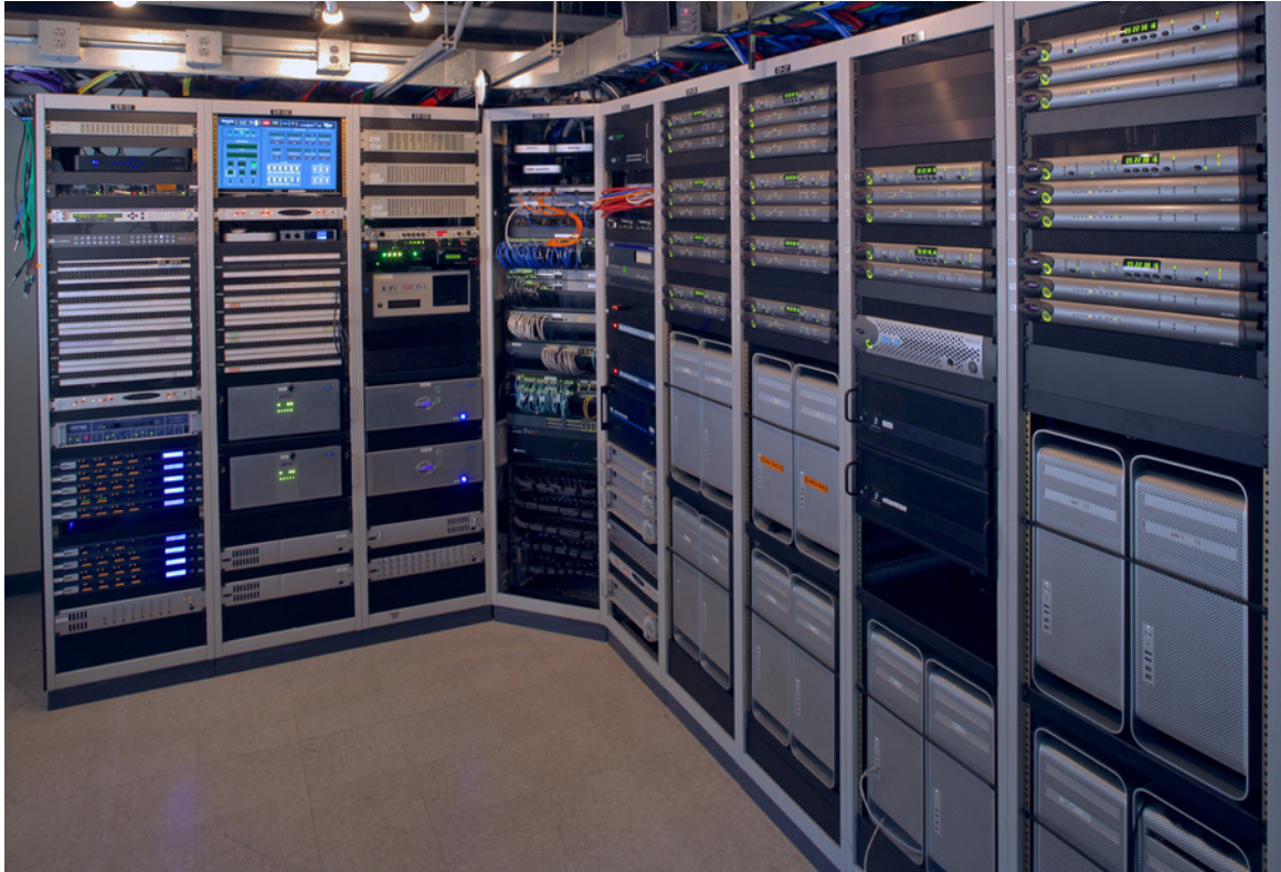
STAGE A MACHINE ROOM
